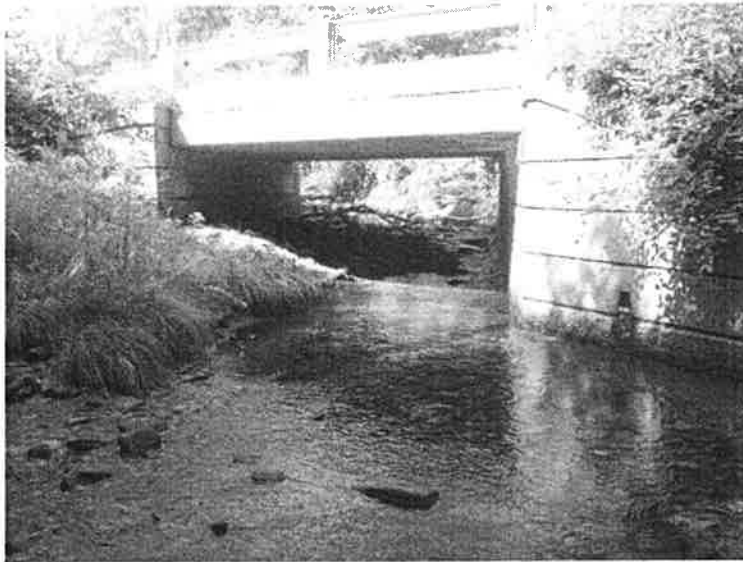
Townsend Road bridge over the South Branch Saxtons River is a major constriction for the measured bankfull channel width. The bridge is also poorly aligned and the opening is partially filled with sediment, increasing the fluvial erosion hazard risk at the site. 28
