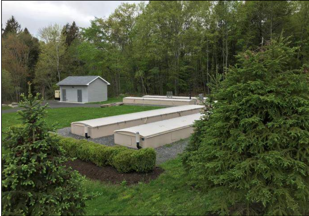
FIGURE 6.4 Orenco Advantex PBF System in Hyde Park, NY
