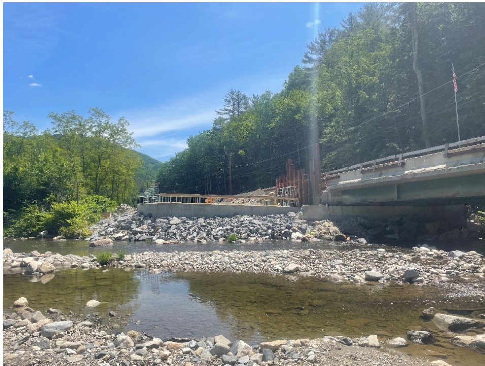
Crews complete the installation of the second bridge abutment and stone fill along the Saxton River's edge.
