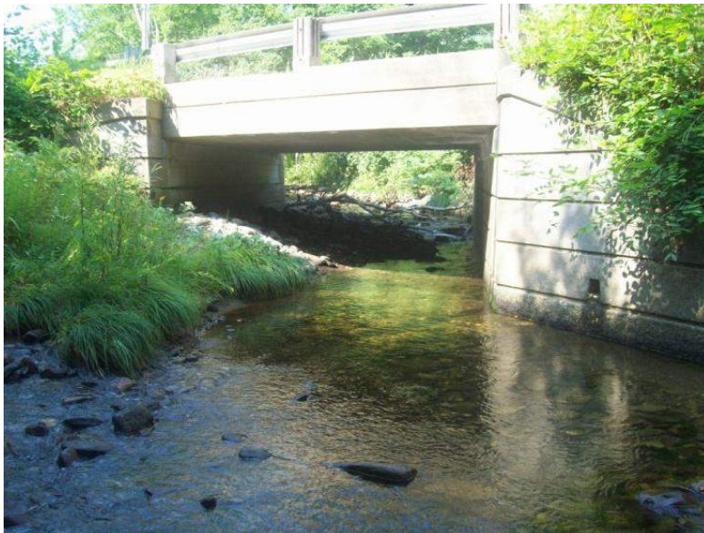
Townsend Road bridge over the South Branch Saxtons River is a major constriction for the measured bankfull channel width. The bridge is also poorly aligned and the opening is partially filled with sediment, increasing the fluvial erosion hazard risk at the site. 28
